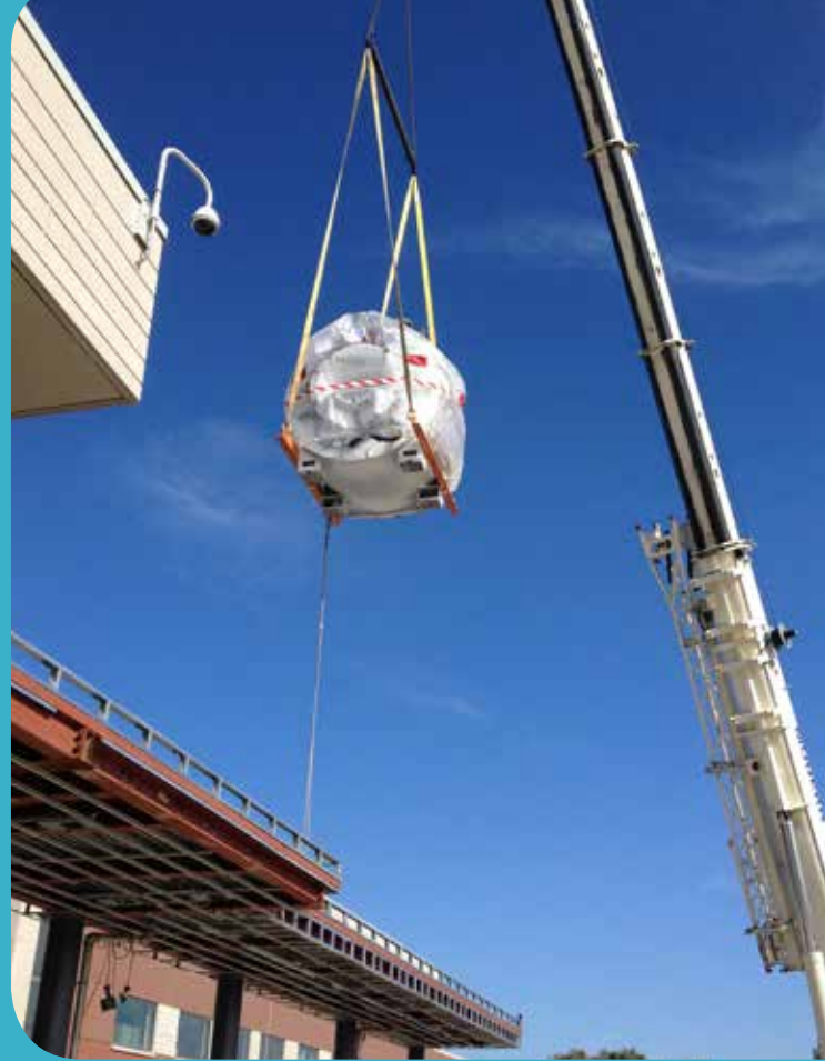
The MRI was lowered into a temporary shaft, just outside the Main Entrance to the new building, off of West 5th Street.
